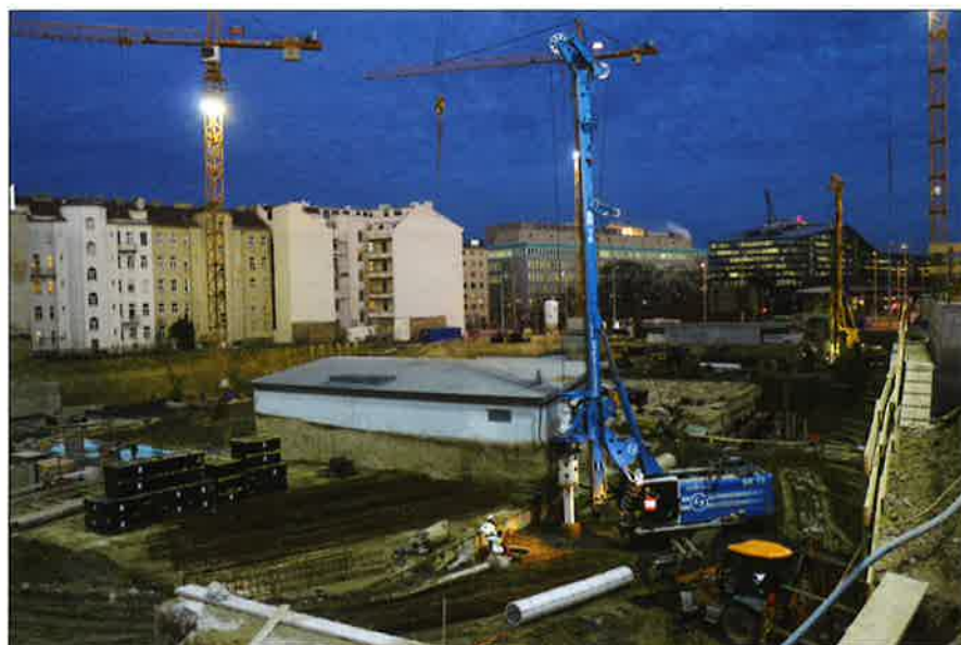
Side view of the job site area. Six tower cranes are installed around the entire perimeter as support machines
