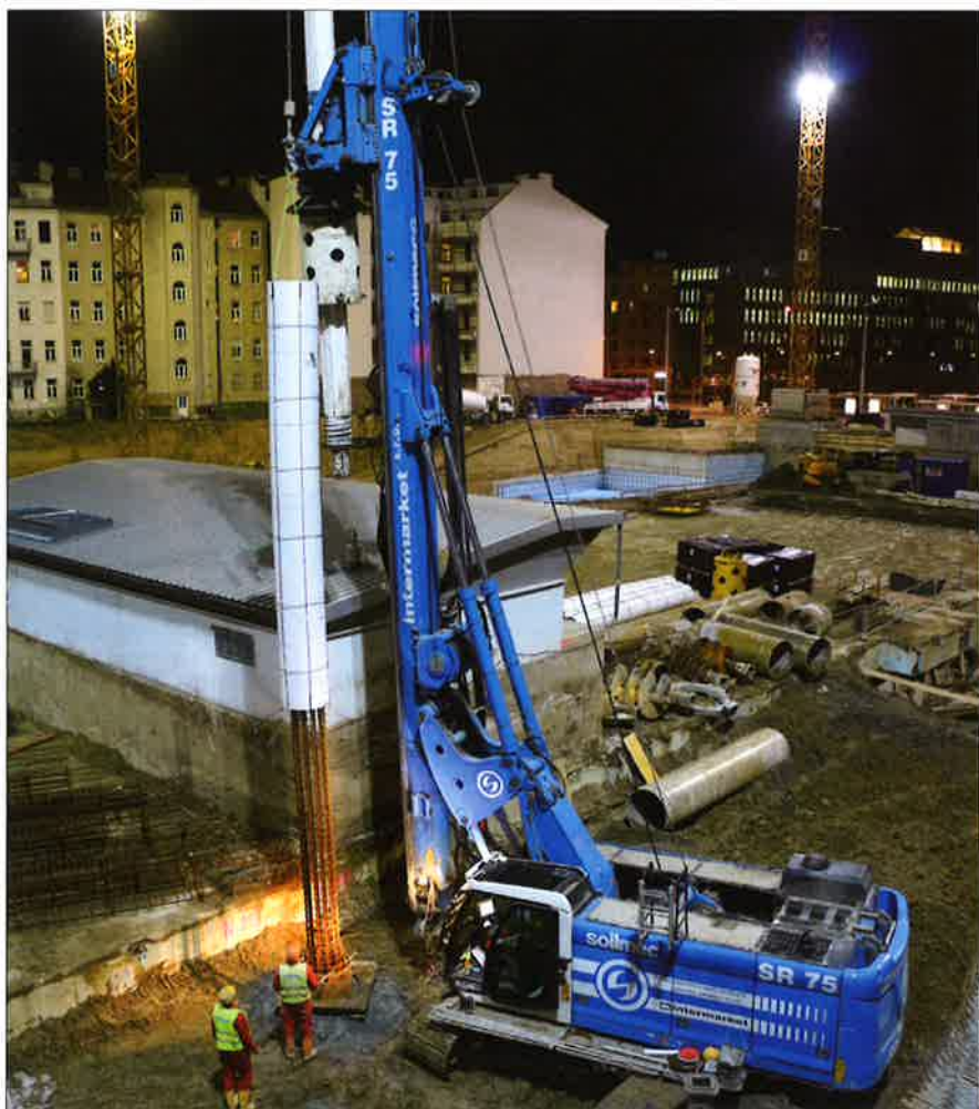
The special cage used for all the piles near the train cut-off wall structure
