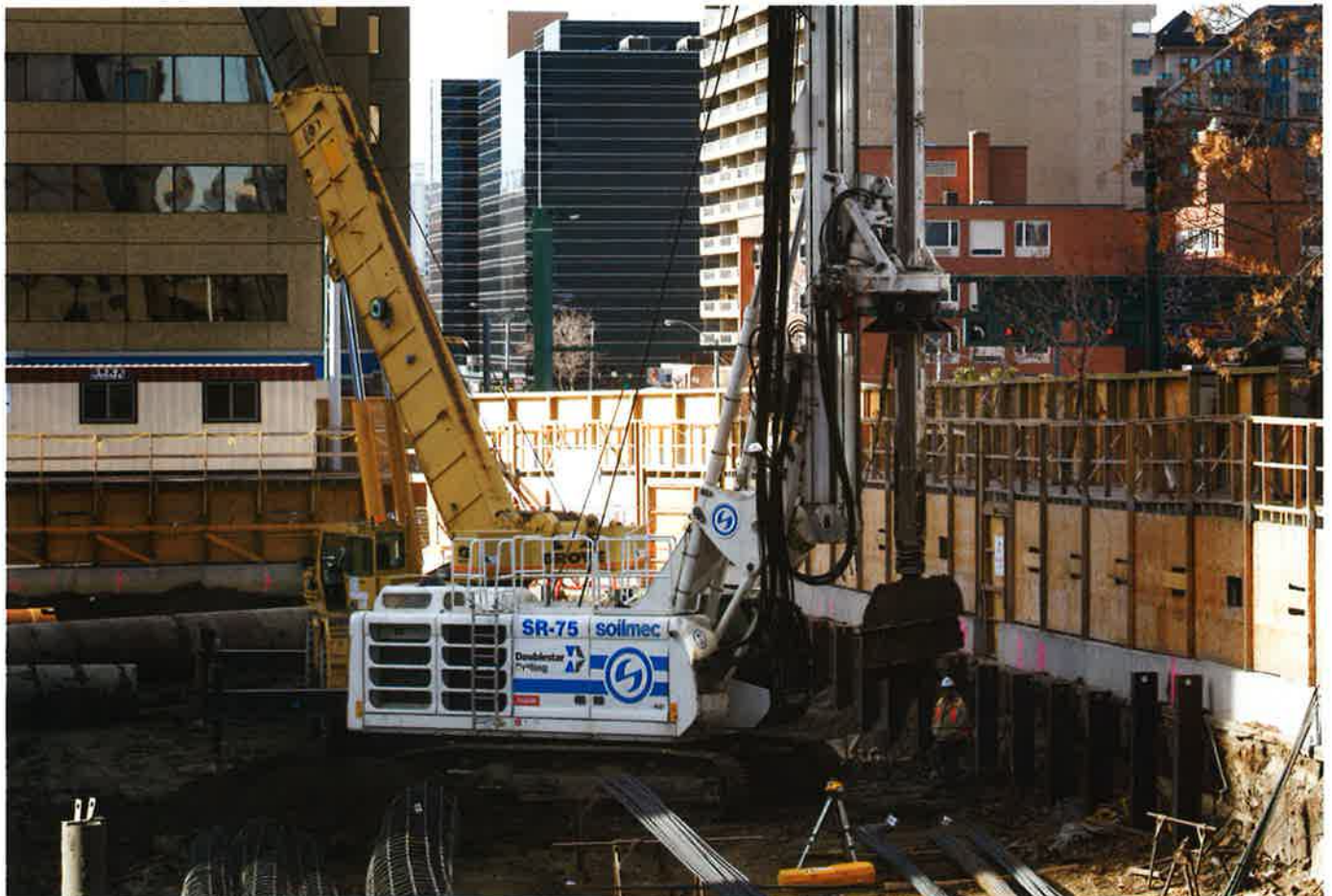
Doublestar Drilling using their Soilmec SR75; Doublestar has a large range of heavier drills over 150,000 lbs
