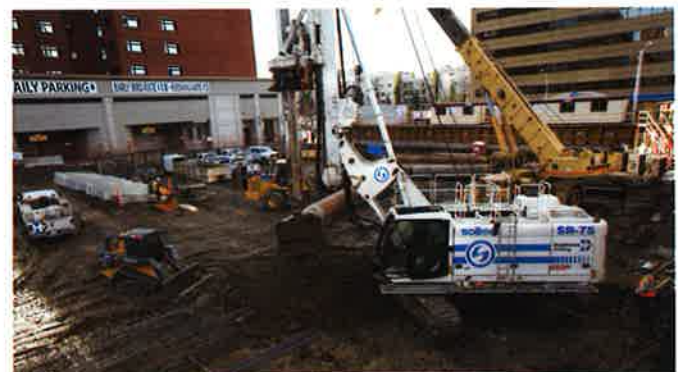
Doublestar Drilling completing large piles above the Edmonton LRT on Jasper Avenue
