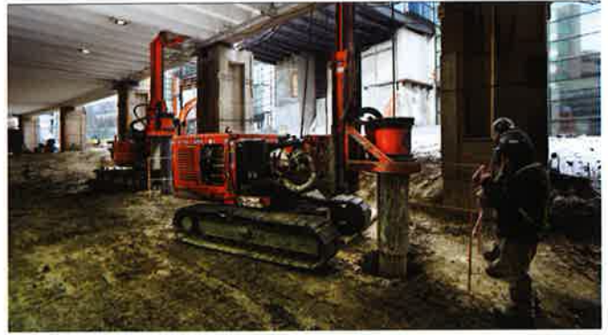
Doublestar Drilling completing four-metre rock socket piles in only 14 feet of headroom at the Calgary international airport
