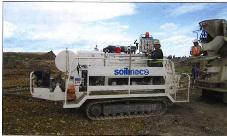
Keller Canada managed the congested job site using two Soilmec P6.90 concrete pumps
